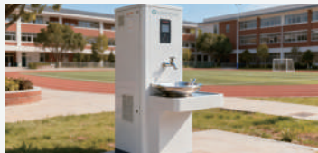
Public Direct Drinking Water & Pipeline Systems
