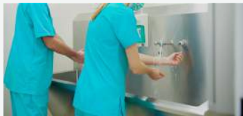
Hospital General Water Systems
